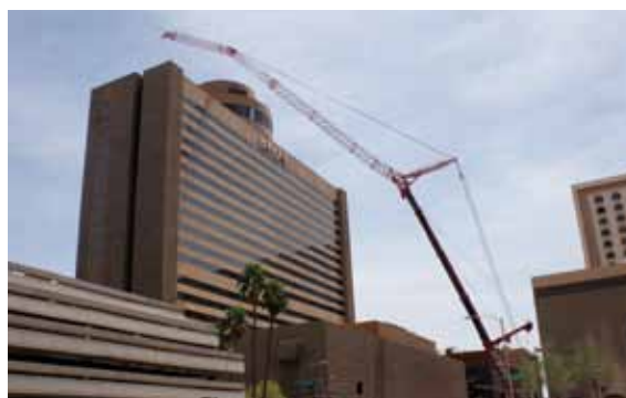
SWIR's largest crane on the job at the Hyatt in downtown Phoenix
